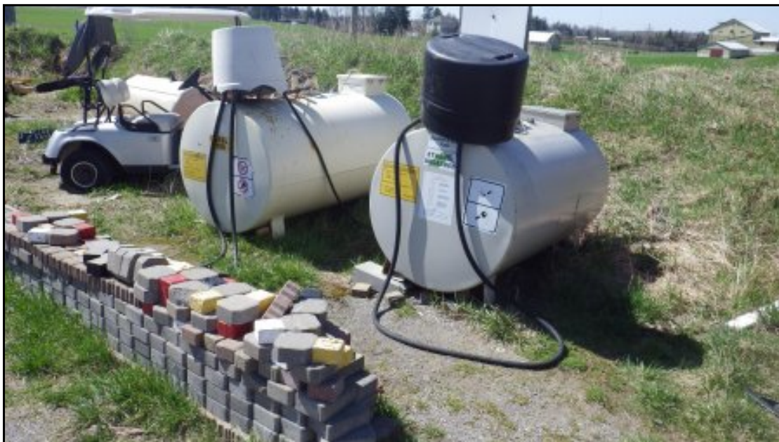
Gasoline and diesel ASTs with no secondary containment at 100 Wilmot Line situated west of the Maintenance Building, facing west.
