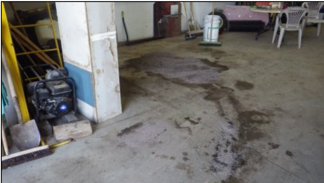
Staining observed within the Maintenance Building at 100 Wilmot Line.
