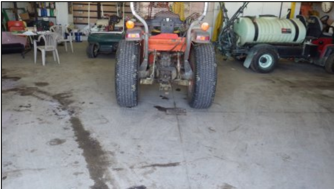
Observed staining near the drain in the Maintenance Building at 100 Wilmot Line.
