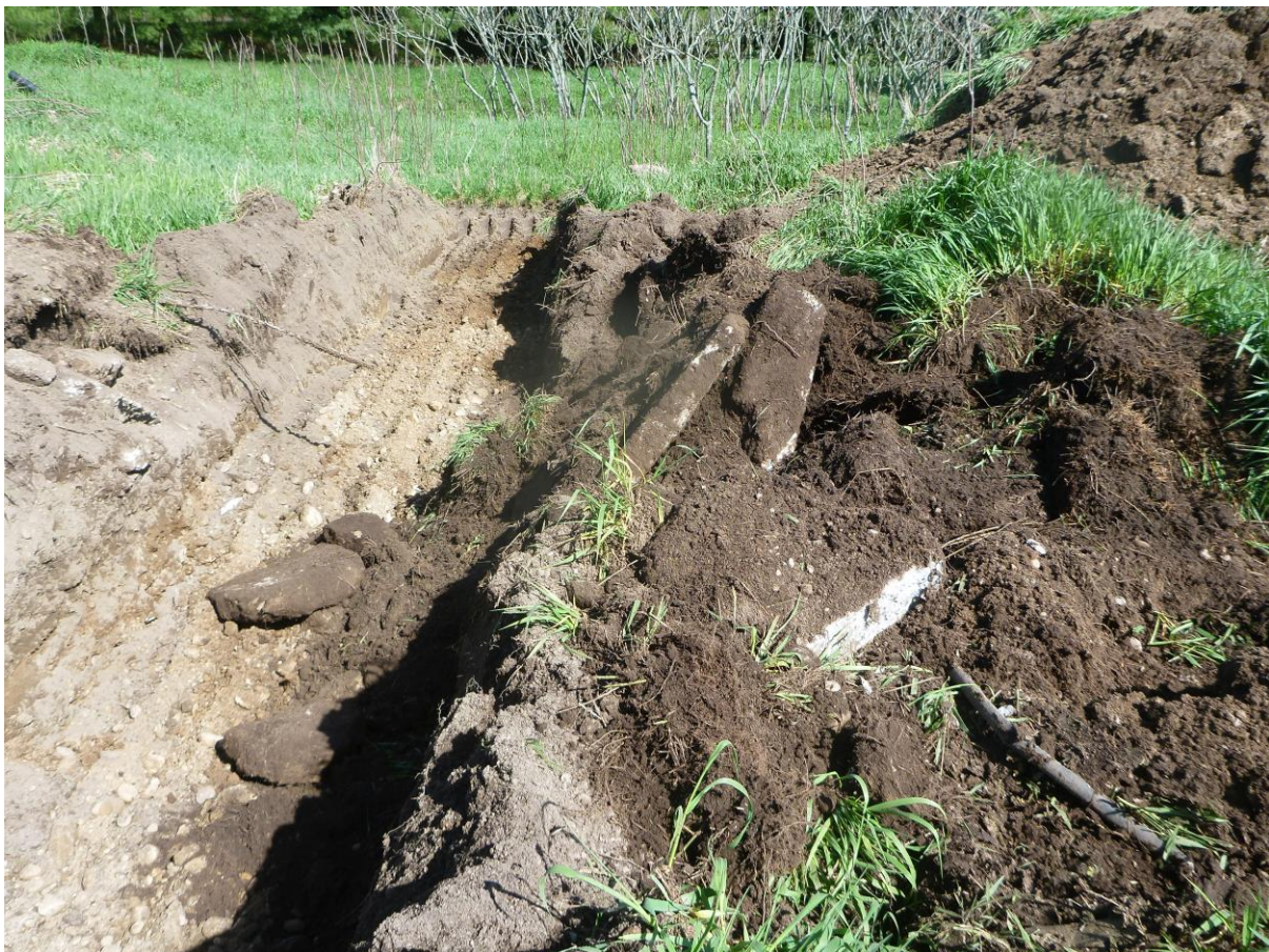
Photograph 4: View of construction debris in excavated fill material of TP2
