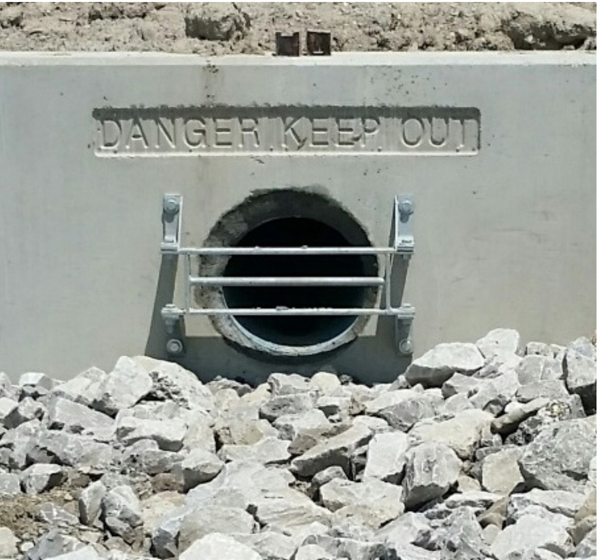
5 Sewer Safety Grate
