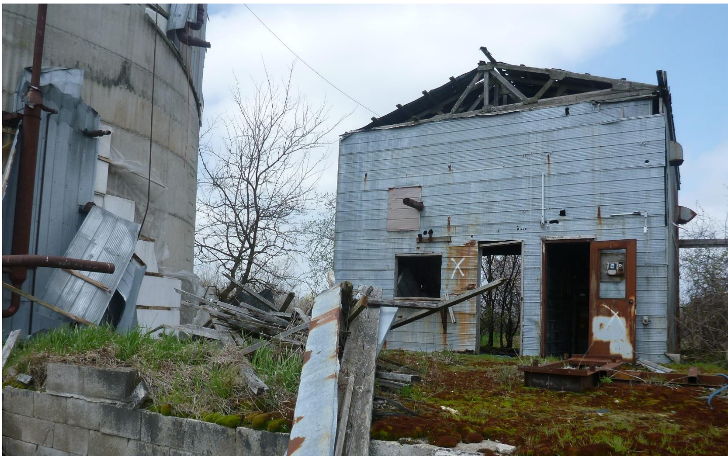
Photograph 10: View of the derelict digester facility.
