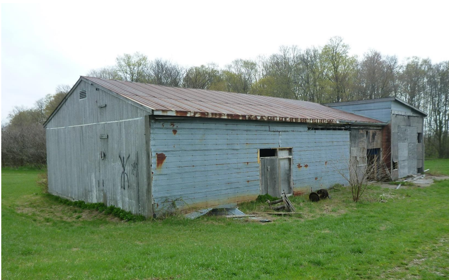
Photograph 7: View of the derelict maintenance shop building on the south end of the Site.
