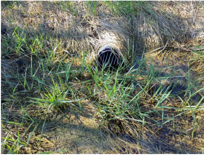
Photo 7. Tile drain outlet.
